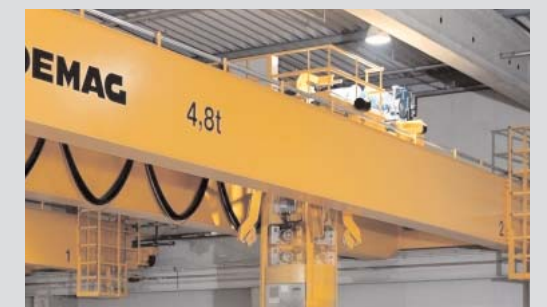
For gantry crane position determination (BPS 8 and BPS 34/37)
